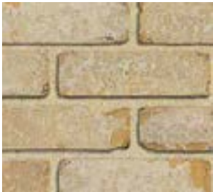
Mid buff brick with matching mortar
